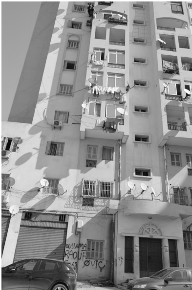
Figure 12. A typical example of alterations to the balcony
