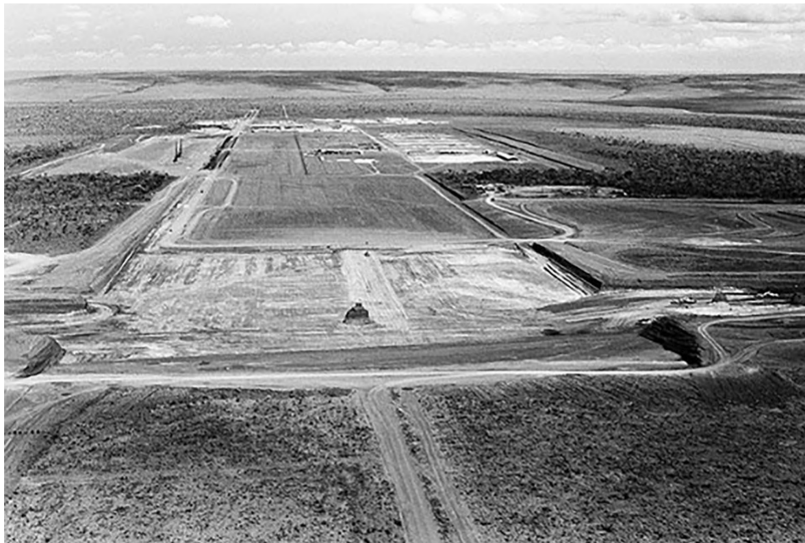
fig. 8. Brasília, Ground Zero, Blus Platform and Esplanade of Ministries under construction, October 1958, Photo: Mário Fontenelle (Arquivo Público do Distrito Federal)
