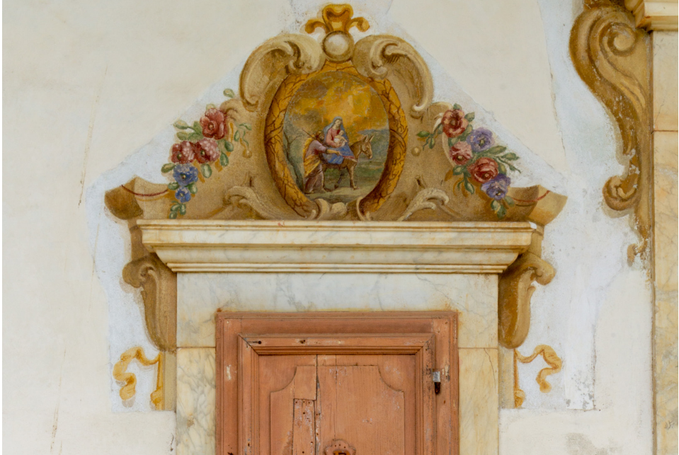
Fig. 7 – Painting on the top of the small door used to bring food to the monks, preserving their isolation (north arm, “P” cell). Differences in colour and grain are visible between the paint closest plaster and the surrounding portion (photo by the authors, March 2019).
